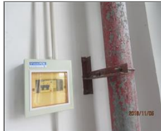
External photo(s) of the production unit(s) Finding 7.13 No warning sign.JPG
